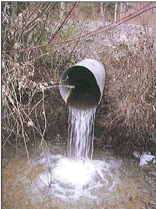
Photo 2: This 2 foot (shotgun) culvert conveys and supplies intermittent hydrology into the identified wetlands. There is a 3 foot vertical drop at this culvert outlet. In terms of potential fish habitat, this culvert represents the end of the road along this stream channel.
