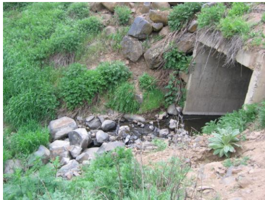
Figure 50. STC-1. Box culvert barrier
