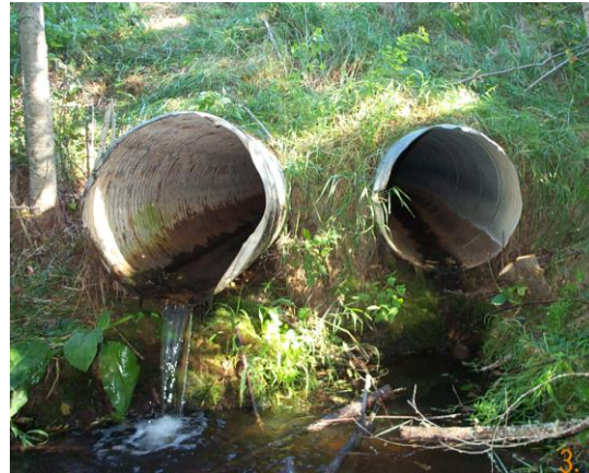
Figure 5. Multiple perched culverts
