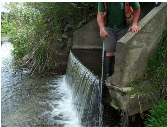
Figure 6. Perched box culvert and sheet flow
