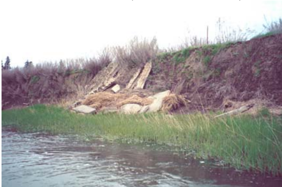
9.1 Right bank erosion and fill material
