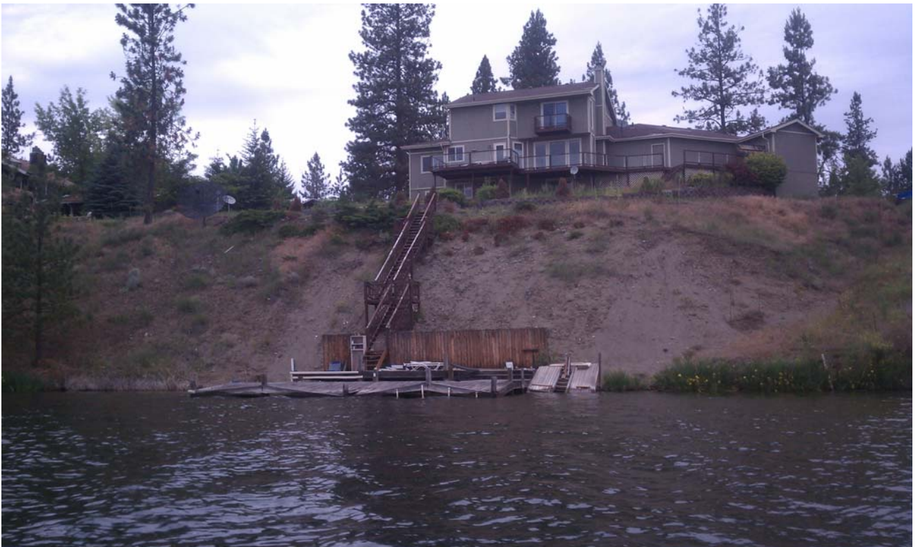
Unstable slope between house and dock, dock failure
