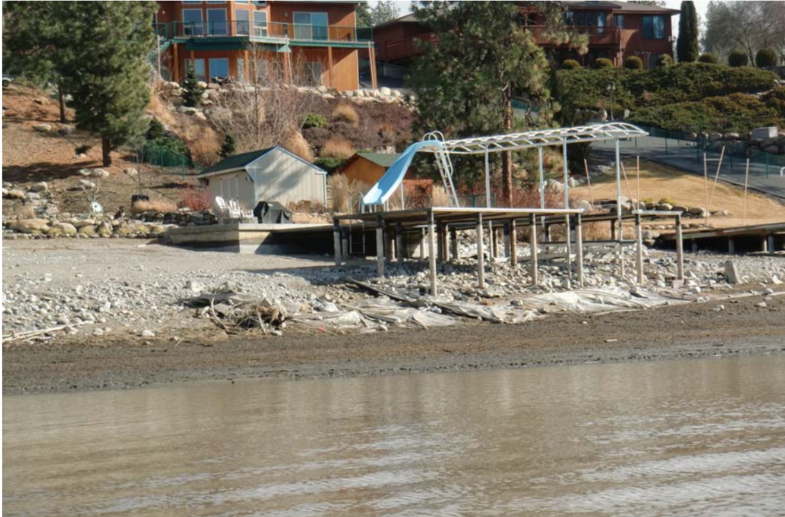
Poorly installed bottom barriers
